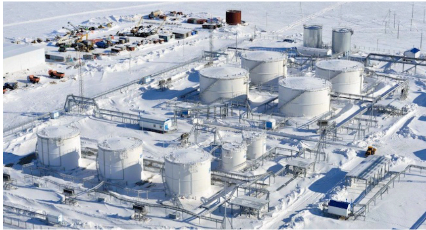
The Sabetta facility being built on the Yamal Peninsula will allow LNG exports from 2017 onwards. Novatek
