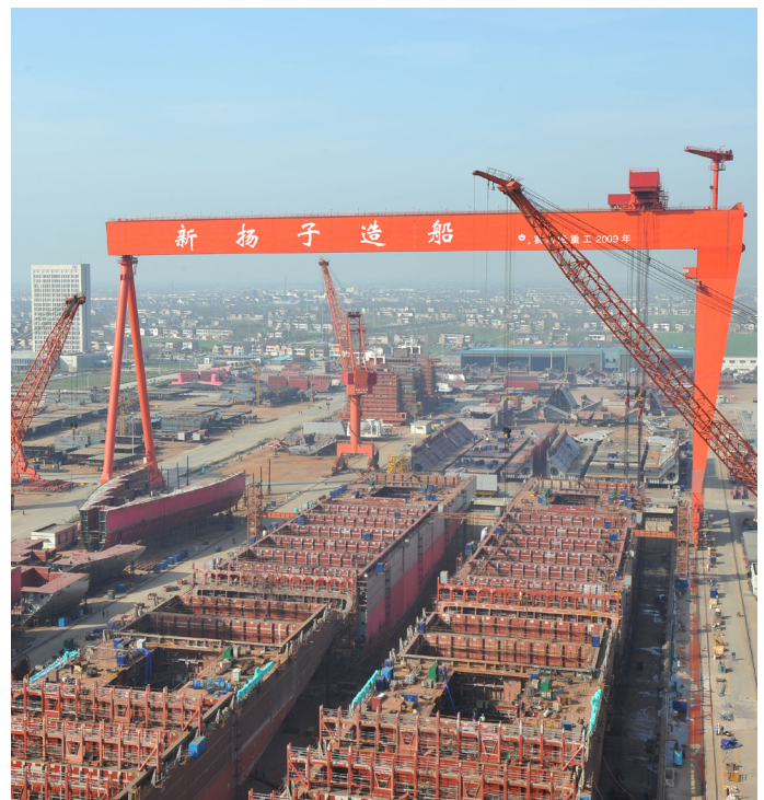
Yangzijiang Shipbuilding has been preparing for the construction of LNG carriers for some time, says chairman Ren Yuanlin.
