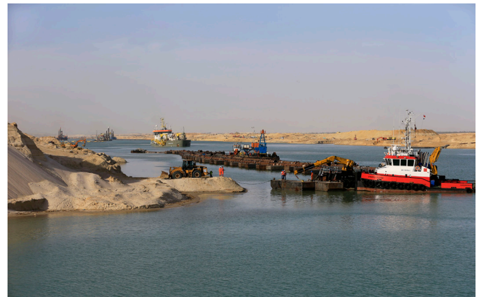
Under construction: the new Suez Canal channel, due to be completed later this year, will allow ships to travel in both directions simultaneously.
